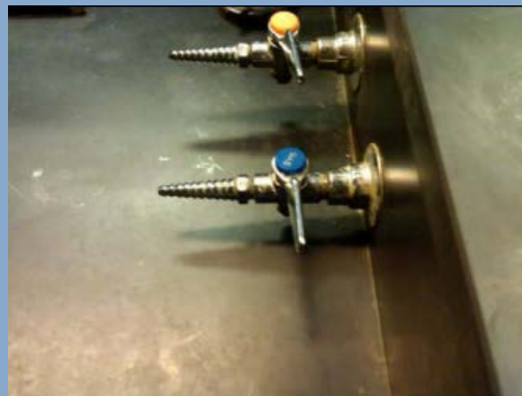
Gas valve stems in the off position
